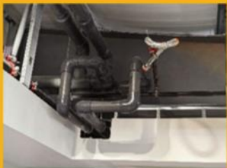
Heat Pump Supply Lines
